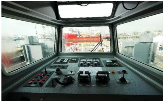
Aft bridge console with remote FiFi controls
