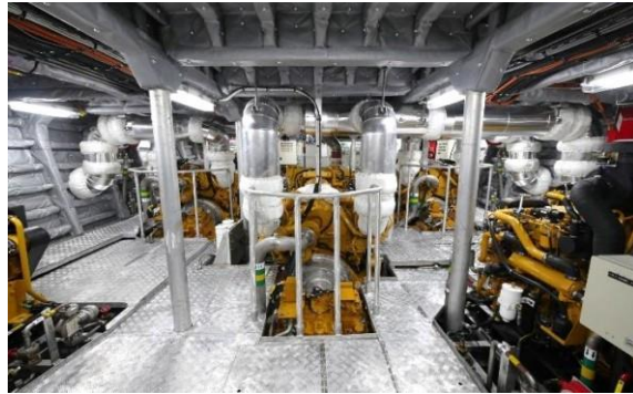
Spacious engine room
